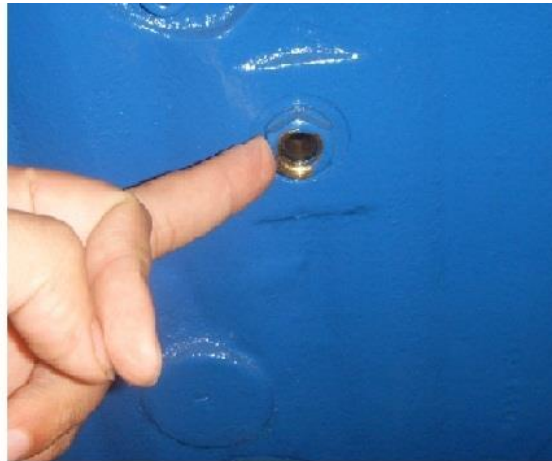
the window on the gearbox
